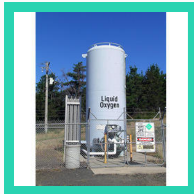
Oxygen Storage Tank
